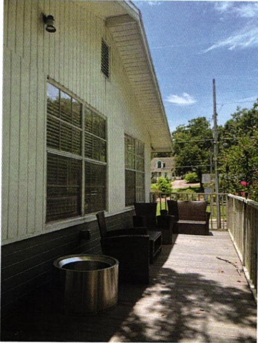
Picture of the side of the home, with the aluminum windows, wood siding, and concrete block. The request is to replace these windows as well and update the siding to a horizontal cement or composite board, painted white.
