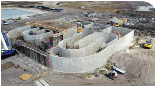
Halff Experience | Gibson Place Utilities Wastewater Treatment Plant
