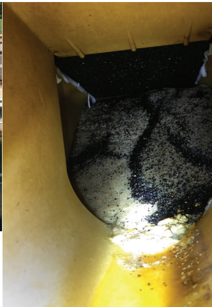
Failed Filter Showing Unwanted Breakthrough of Filter Media
