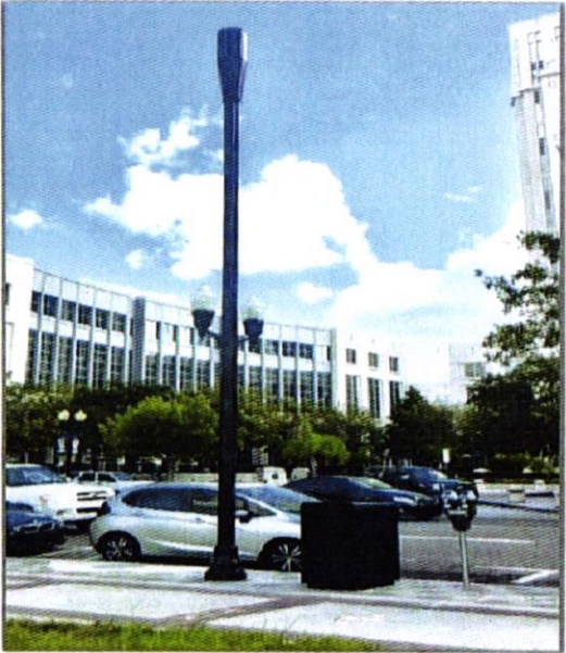
City of Orlando Acorn Light Node/Pole
