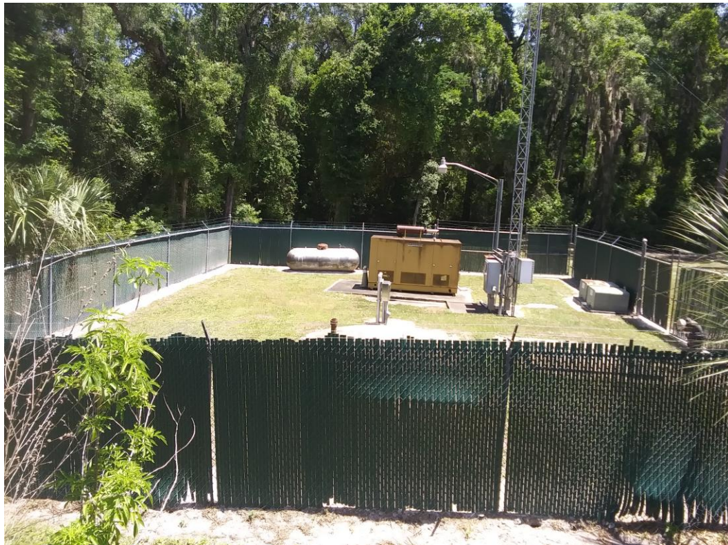
20) City of Mt Dora Forest Preserve – – Closeup of Water Treatment Substation along west side of Lake John
