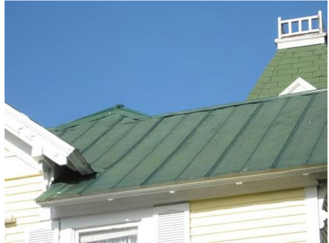
Keep metal roofs painted. (305 South Eighth Street)
